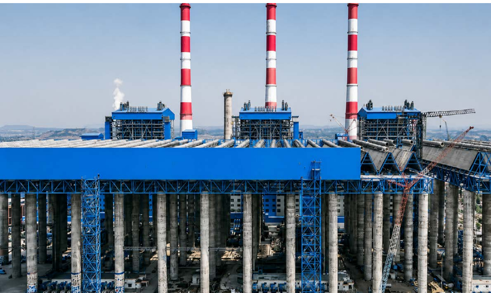
Tandwa Power House Air Cooled Condenser
